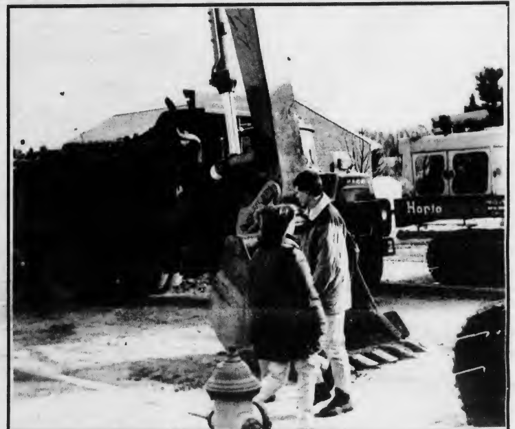
Shawn Hoke/Clarion Call Construction continues at Clarion. The Steamline project is now focusing on the area outside of Marwick Boyd and Becker Hall.
