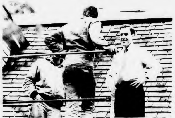
SEN. PAUL HAROLD inspects the new roof being constructed on the Dorothy Quincy Homestead on Butler Rd. The new split cedar shingle Mansard roof is being constructed by Christopher Paine and Richard Paine of A.W. Paine Construction Corp. of Marshfield. Harold had $100,000 added to last year's state budget to fund the new roof. Owned by the MDC, the homestead is maintained by the New England Society of Colonial Dames. The roof repair and restoration should be completed in July.
