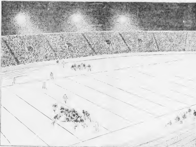
The banks of G-E floodlights at Georgia Tech's Grant Field can be adjusted to illuminate track meets as well as football games.
