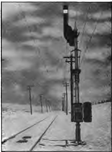
Fig. 88. Illustrating Location of Impedance Bonds in the Track. New York State Rys.
