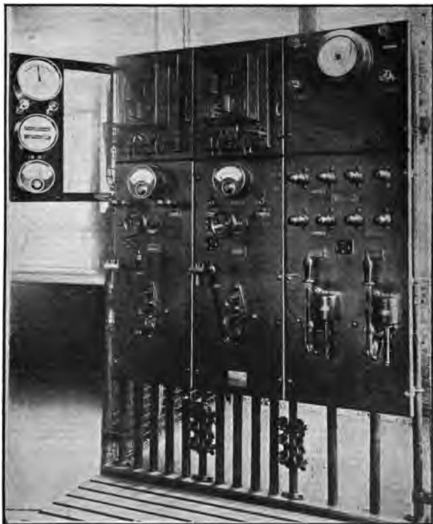
Fig. 191. Main Power House Switchboard Handling Duplicate Generating Sets, Step-up Transformers and Two Sets of Outgoing Mains.
