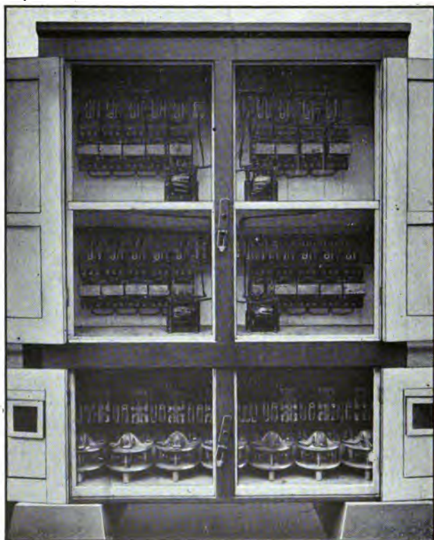
Fig. 134. Detector Track Circuit Impedances, Transformers and Vane Relays. Pittsburgh Division, Pennsylvania R. R.
