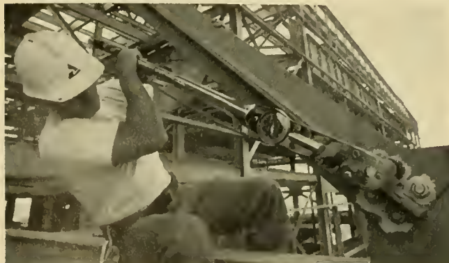
Sitting astride a steel beam, John Dorough, a civil section inspector, torques a bolt to verify the tension.
