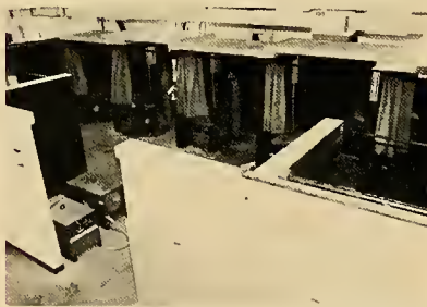
The welding machines are each contained in a curtained booth to protect passersby from flying sparks or eye damage.
