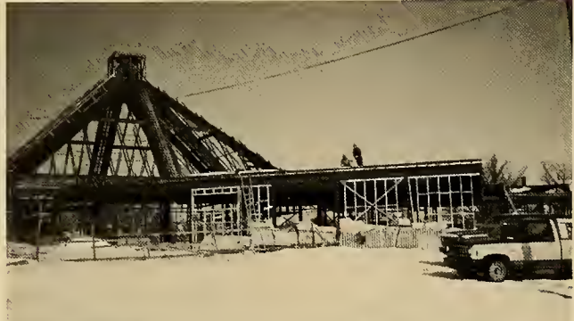
A wood-and-steel-framed St. Ann's church building is under construction in Cape Breton, Sydney, N.S.
