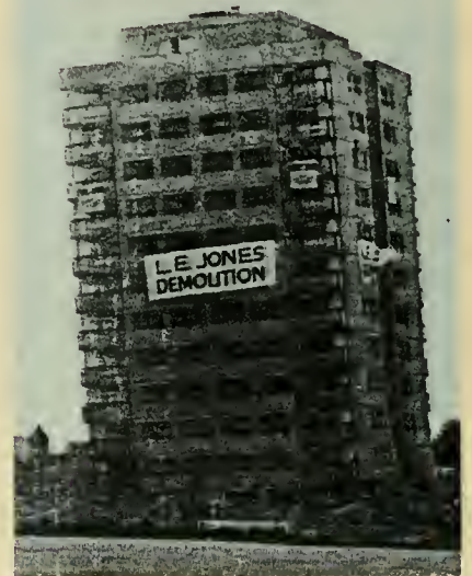
The top 12 floors of the East London apartment building, leaning like the Tower of Pisa but still intact.
