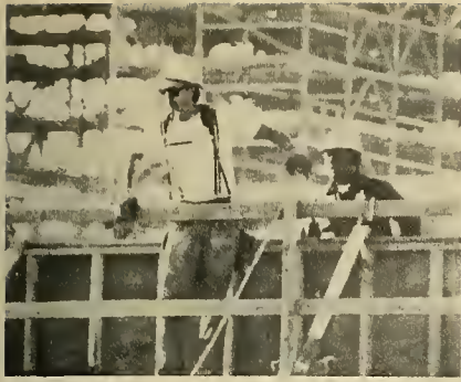
In addition to all of the scaffolding on the project, Carpenters installed the form work for 490,000 cubic yards of concrete. By May 1986 the project was 96% complete.
