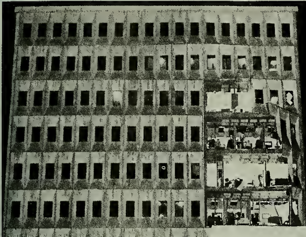
The Parkview Tower office building in Nashville, Tenn., recently suffered damage. An outer wall gave way during a rainstorm, injuring none but leaving the occupants thunderstruck and exposed to the weather. The building, we are told, was built non-union.—Nashville Banner Photograph.
