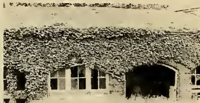
The overgrown vines and broken windows of the carpentry shed show the condition most buildings on Ellis Island were in prior to the restoration.
