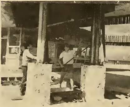
VOC Chairman Mike Decker and State Organizer Gordon Long work on the demolition of the old facade.
