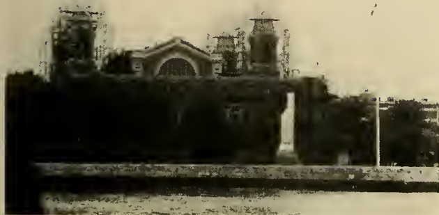
The restoration of the four ornate copper domes and cornices of the main building on Ellis Island presents challenges, especially in duplicating the original ornamental work.
