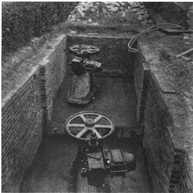
TWO 48-IN. ELECTRICALLY OPERATED VALVES IN VAULT.
