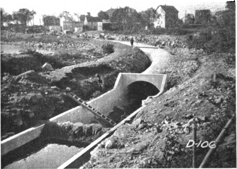
FIG. 1 — JUNCTION OF 10 FT. OPEN AND CLOSED SECTIONS. FALL RIVER INTERCEPTING DRAIN — OCTOBER, 1915.
