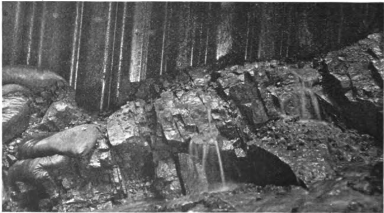
BOTTOM OF DEEP CORE-WALL TRENCH. Good Contact between Steel Piling and Rock.
