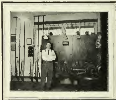
The 4,000-volt distributing switchboard, the oil switches being mounted on the left. At the left are the high-tension levers. (Redwood Station)
