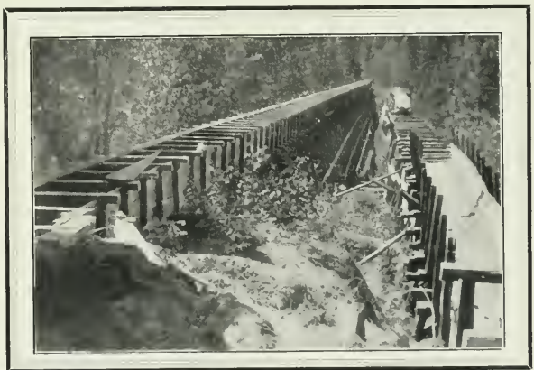
A New Section of Flume Replacing the Old One, Shown on the Right
