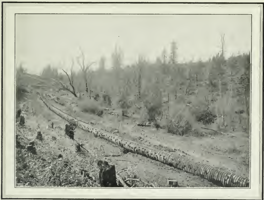
The Stave Pipe-Line from Lake Frances to Colgate
