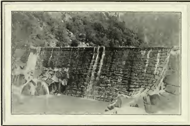
The River Dam As It Looks Today with Its Heavy Facing of Granite
