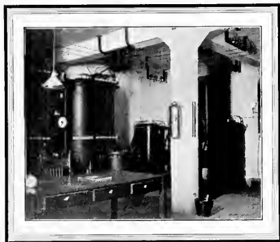
Two of the three 100-kilowatt transformers that supply the local service. (Redwood Station)
