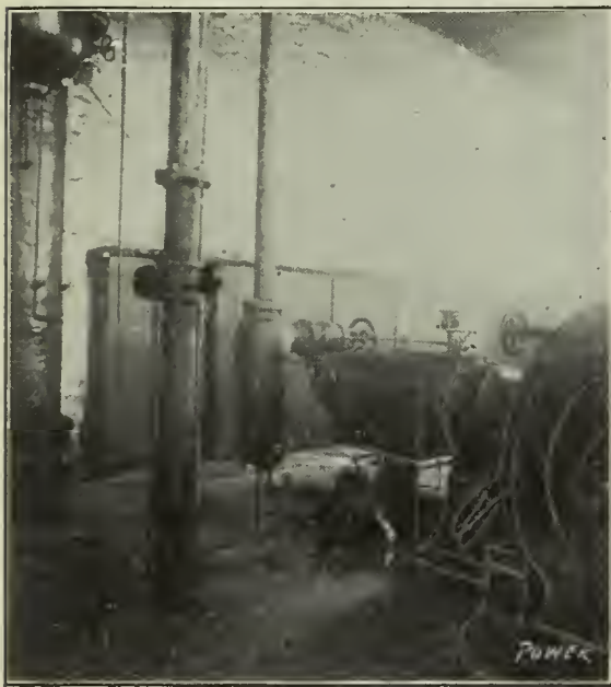
FIG. 3. VALVE AND BLEEDER IN VERTICAL EXHAUST PIPE
