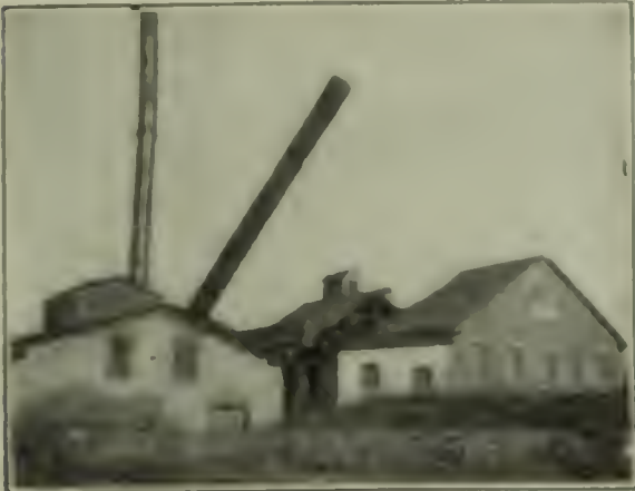
FIG. 1. TILTED IRON STACK
