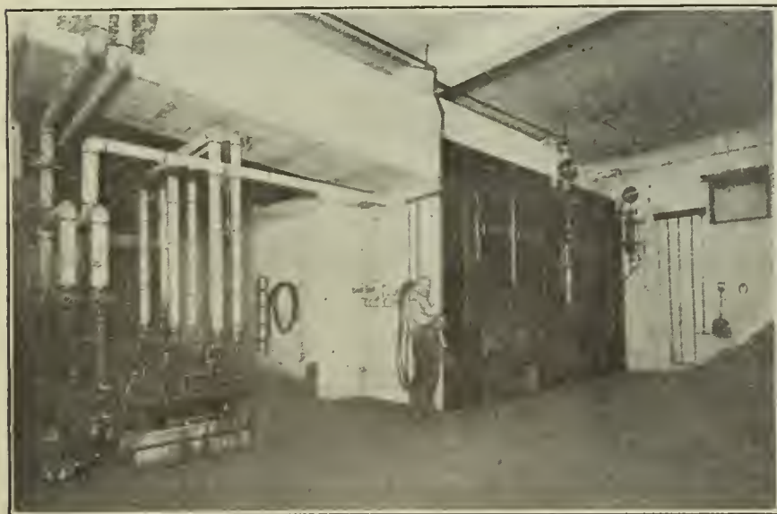
FIG. 1. BOILERS AND FEED PUMPS
