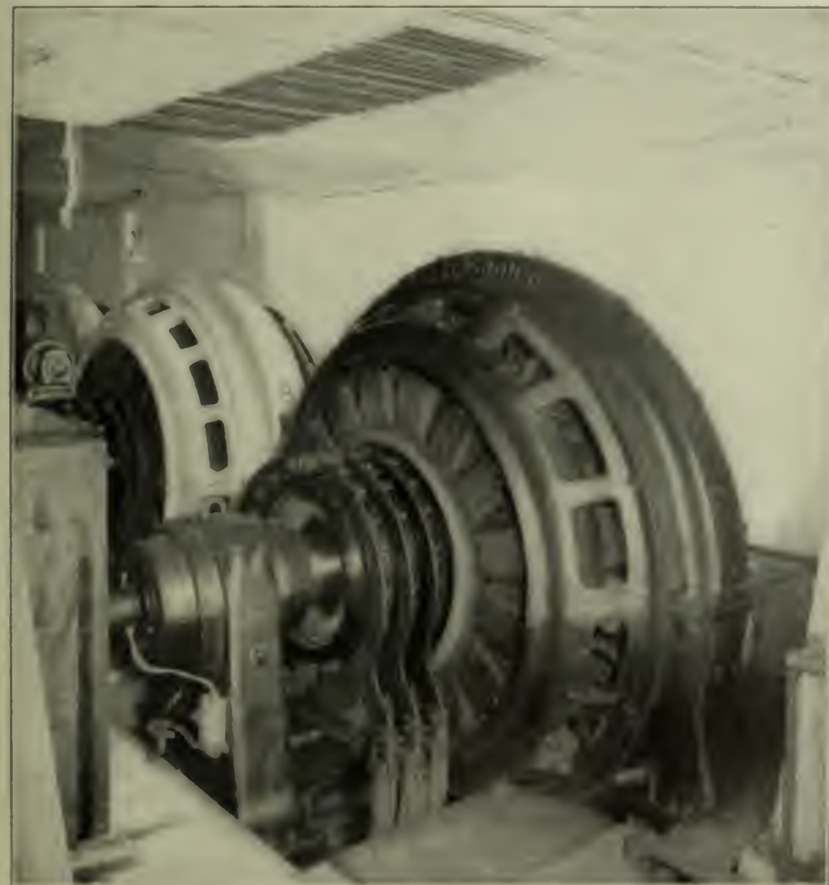
FIG. 6. ONE OF THE SYNCHRONOUS-REGULATOR CONVERTERS.
