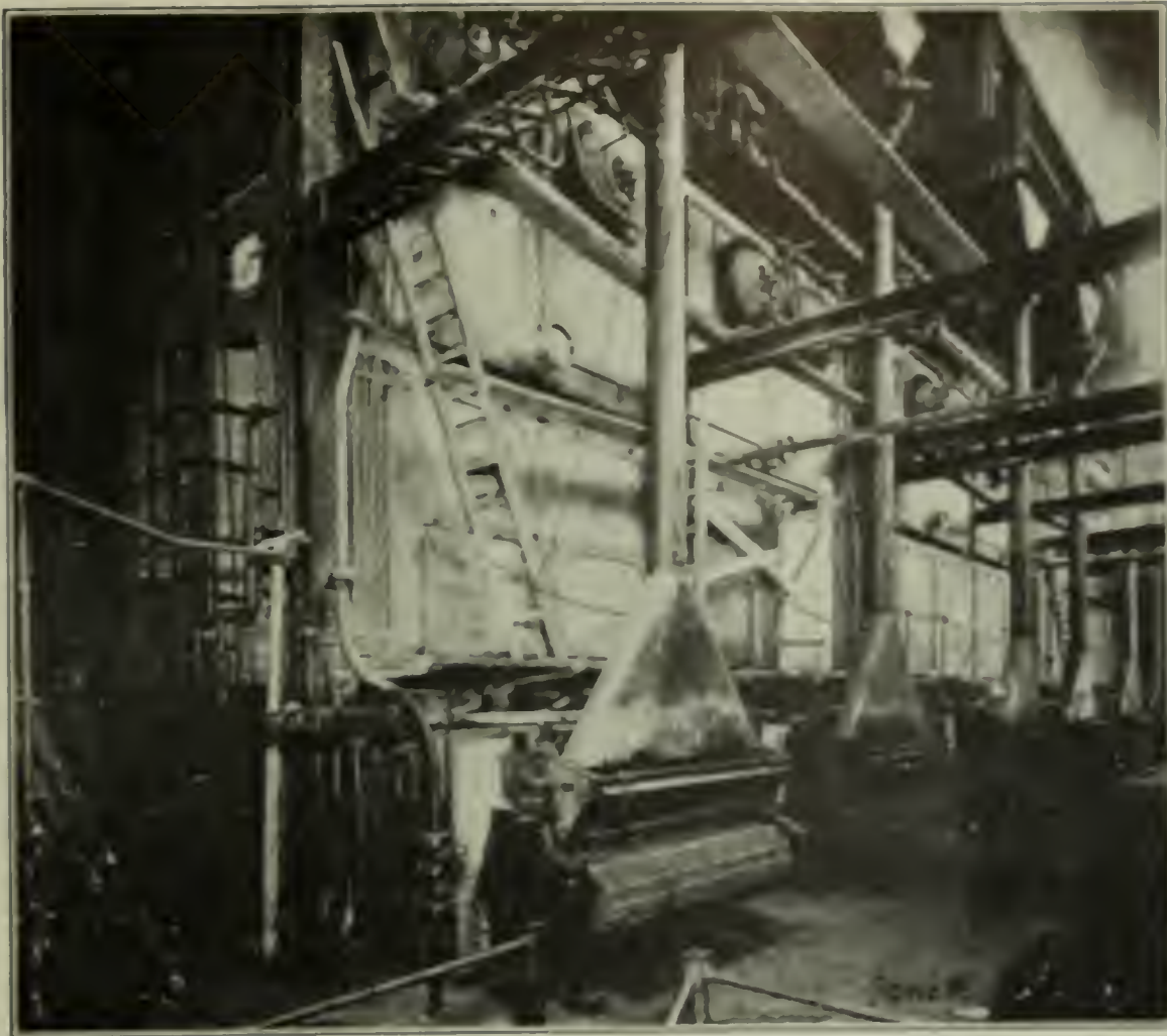
FIG. 6. THE BOILER ROOM
