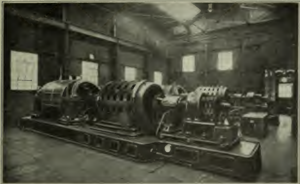
FIG. 1. GENERAL VIEW OF LOW-PRESSURE TURBINES
