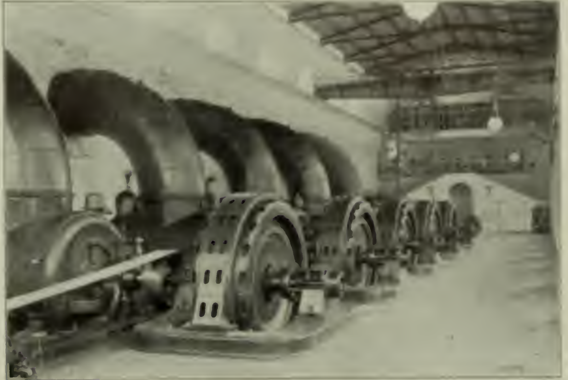
FIG. 3. TURBINE ROOM WITH SWITCHBOARD GALLERY AT ONE END
