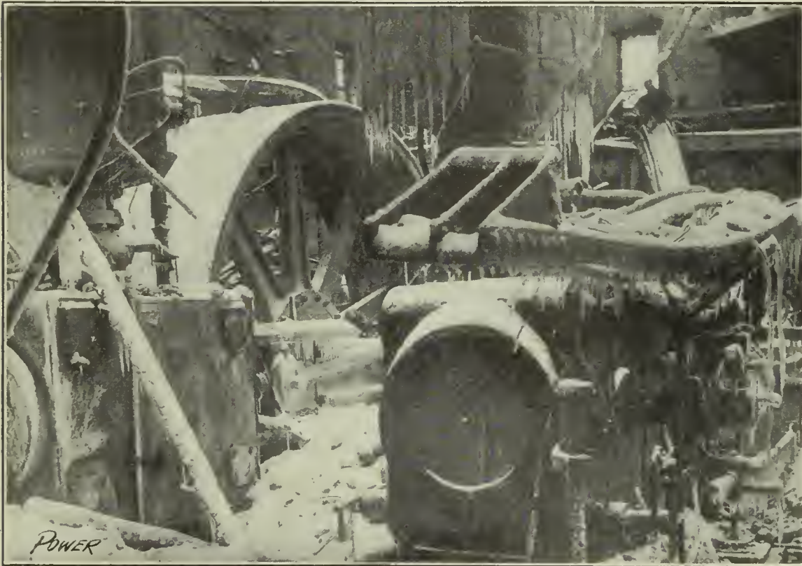
FIG. 1. ONE OF THE CORLISS ENGINE UNITS
