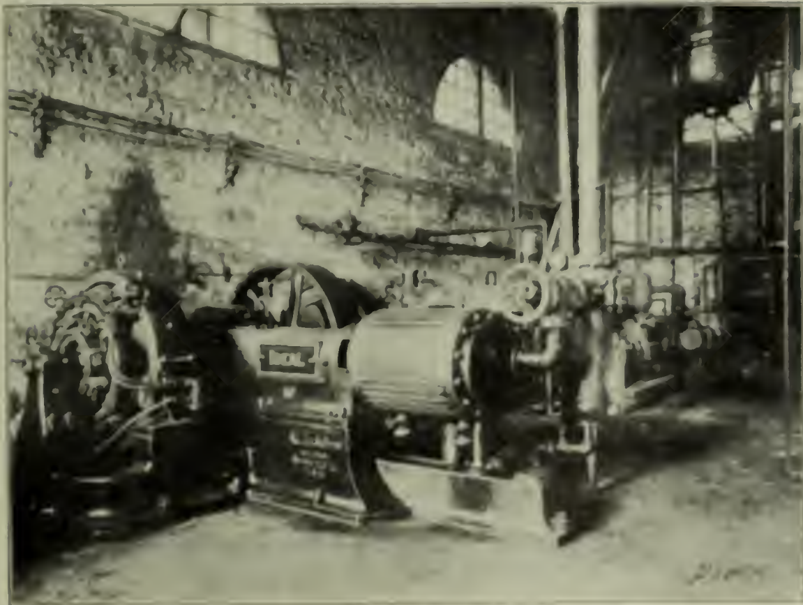
FIG. 1. HOW THE THROTTLE VALVE WAS ATTACHED TO THE STEAM CHEST
