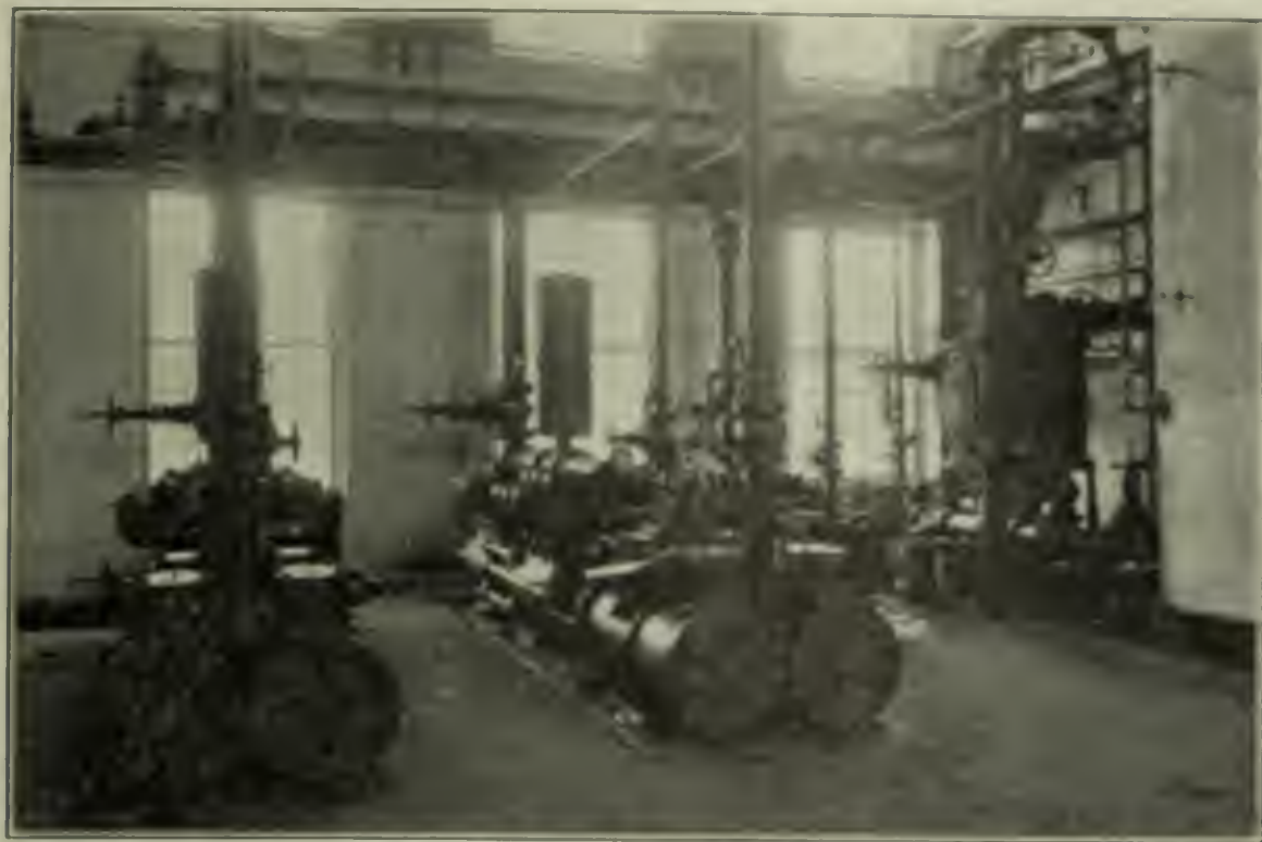
FIG. 8. PARTIAL VIEW OF THE PUMP ROOM
