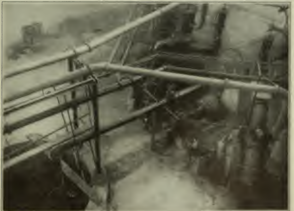
FIG. 9. LOOKING DOWN INTO THE PUMP PIPE
