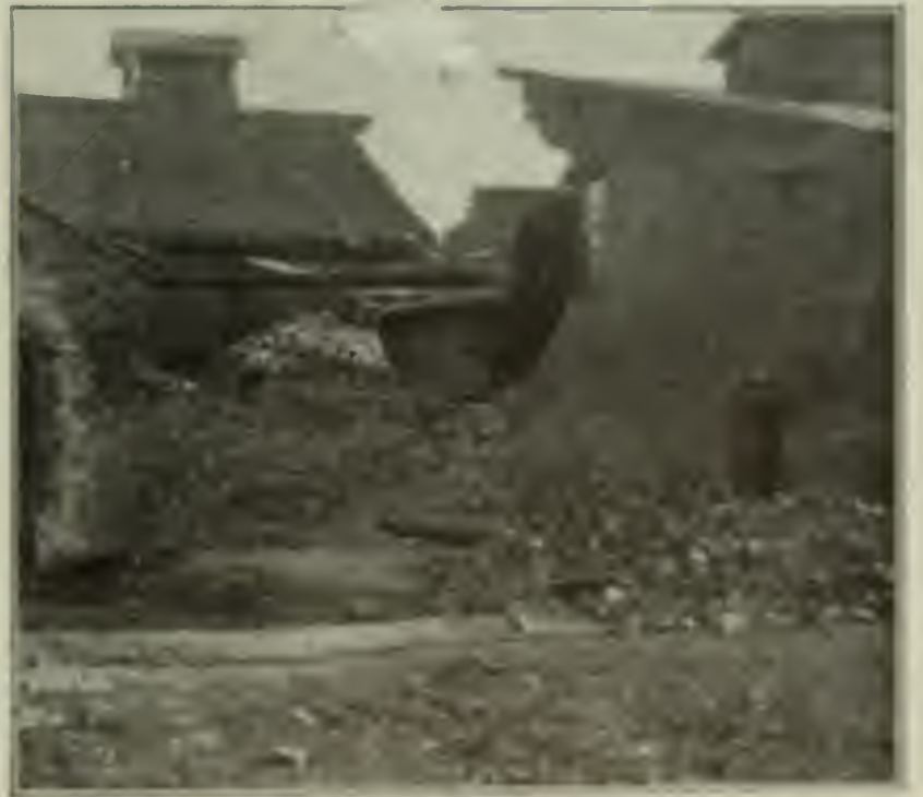
FIG. 3. CRUMBLED STACK BASE AND WRECKED WALL
