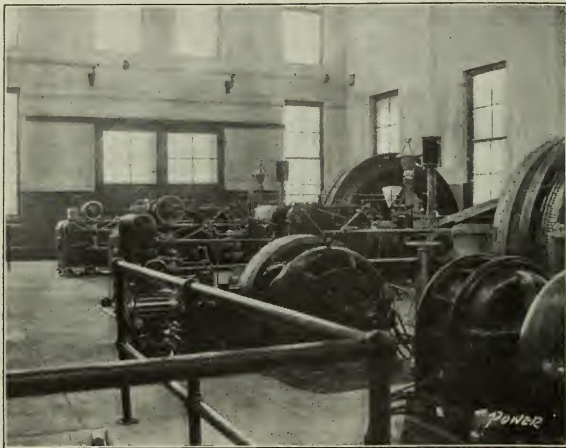
FIG. 4. ANOTHER VIEW OF THE ENGINE ROOM
