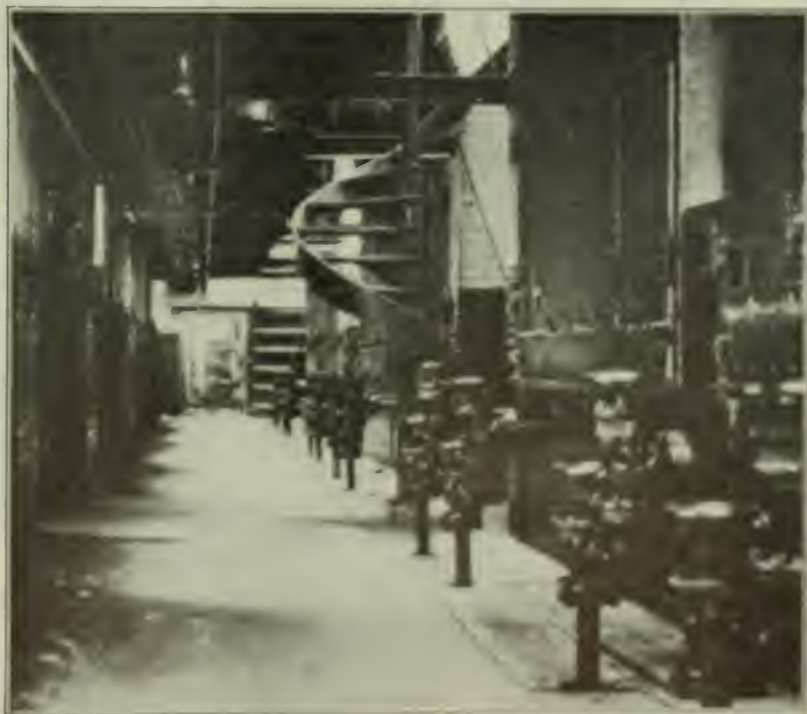
FIG. 4. VIEW BACK OF THE BOILERS.
