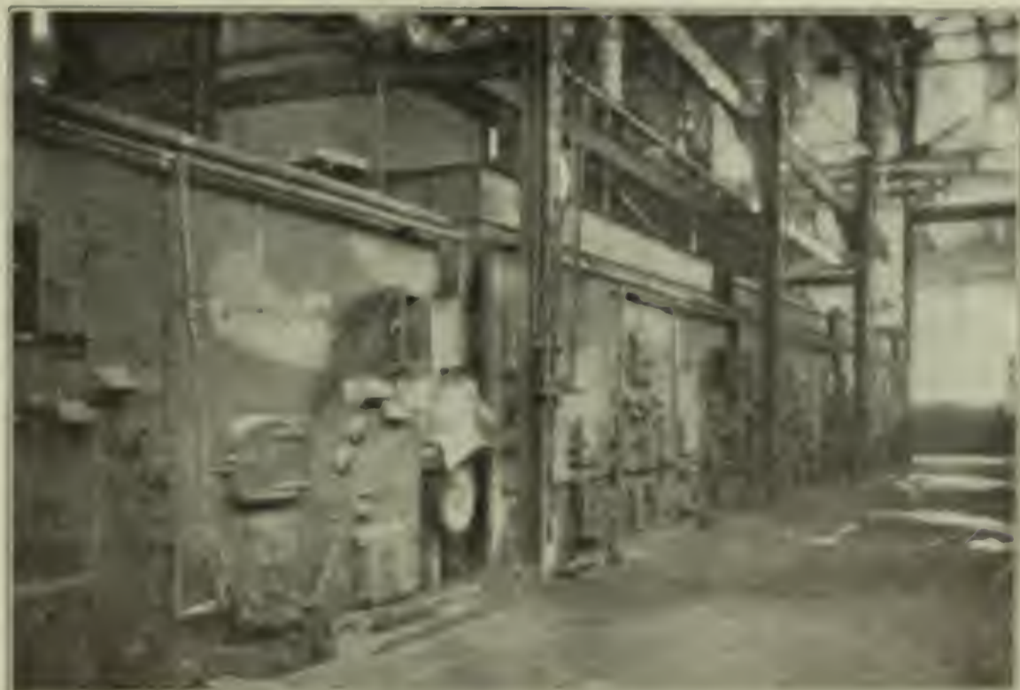
FIG. 3. ARRANGEMENT OF THE FOUR EDGE MOOR BOILERS
