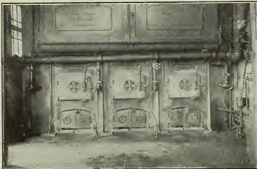
FIG. 2. BURNER IN PLACE READY TO SUPPLY OIL AS A FUEL
