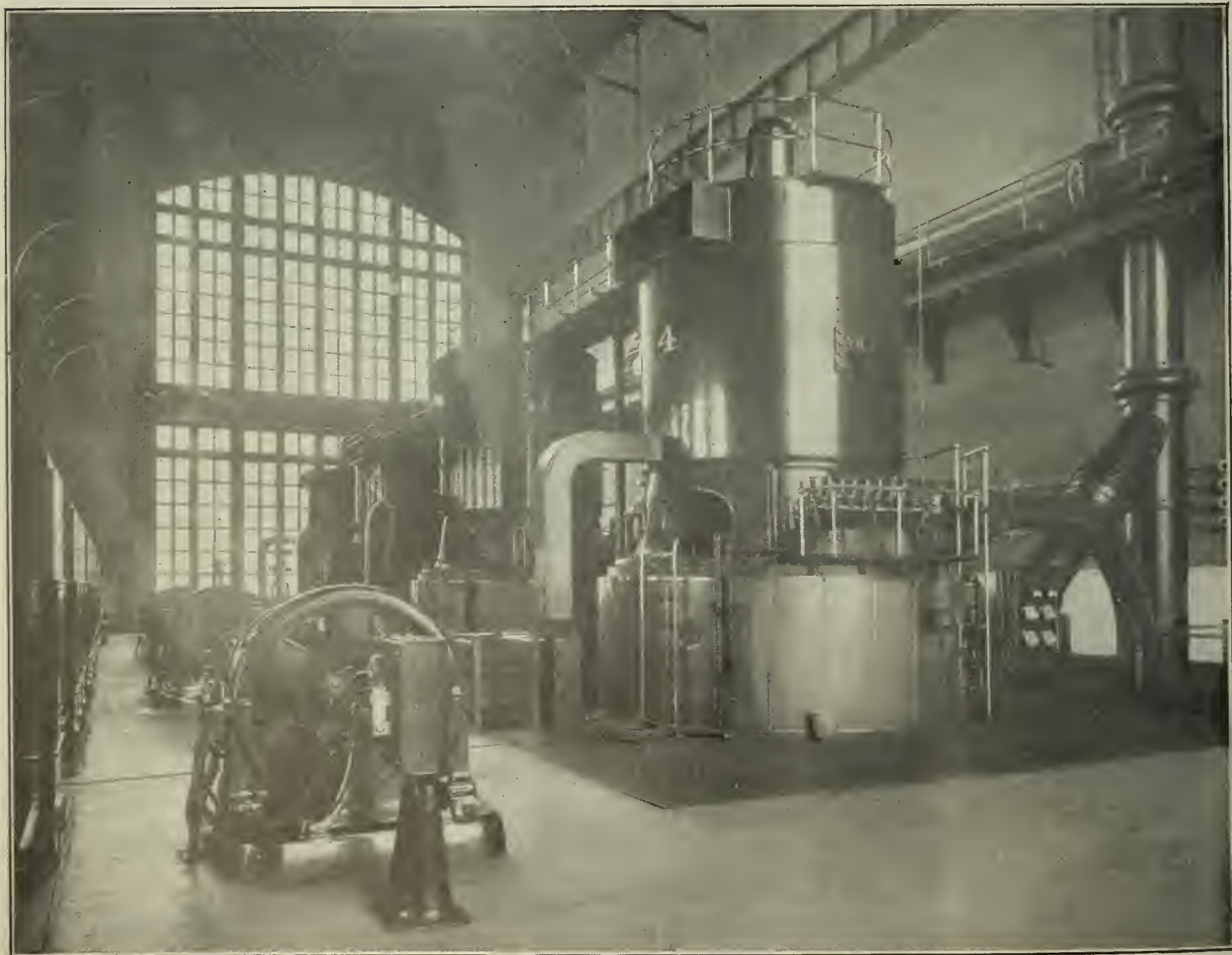
FIG. 1. TURBINE ROOM OF HUDSON-MANHATTAN PLANT
