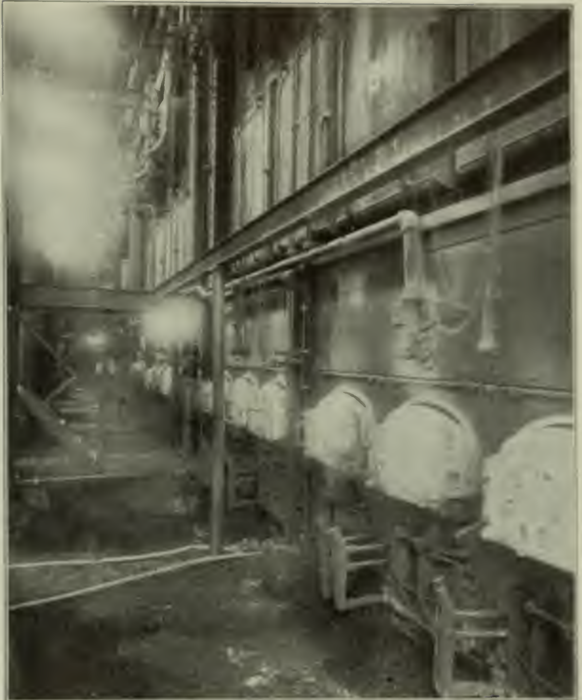
FIG. 2. FRONT OF BOILERS WHICH ARE HAND FIRED
