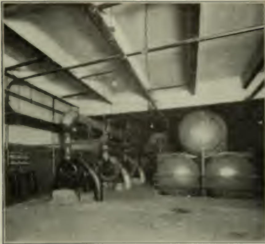
FIG. 5. MAIN HEATING AND CIRCULATING PUMPS
