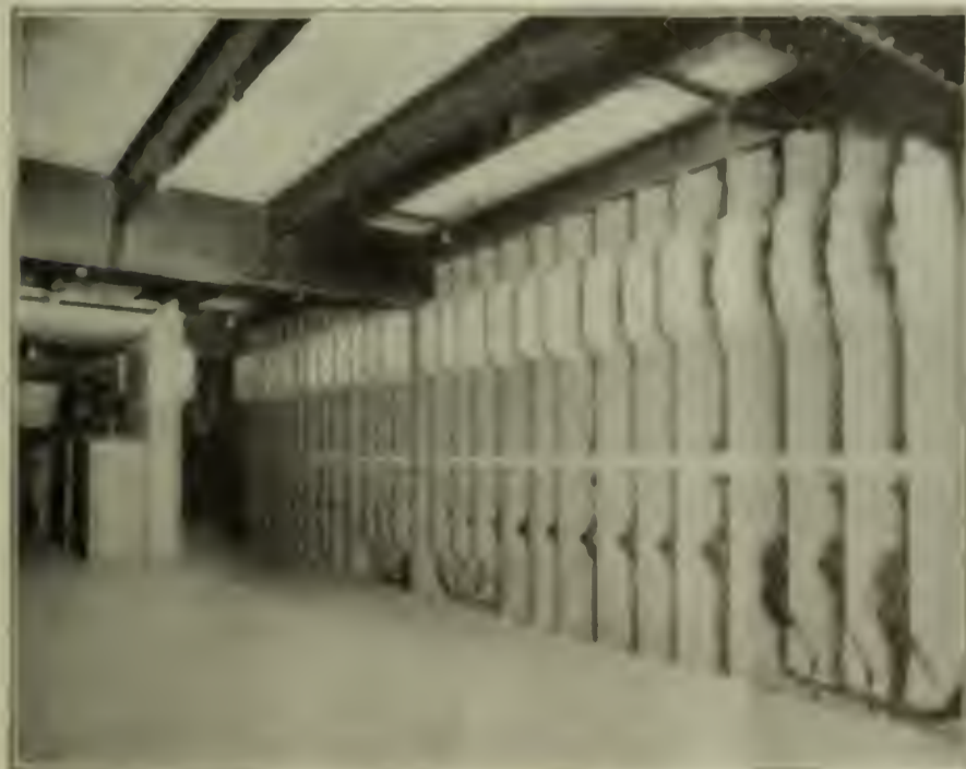
FIG. 9. BARRIS OF HIGH-TENSION SWITCH STRUCTURE
