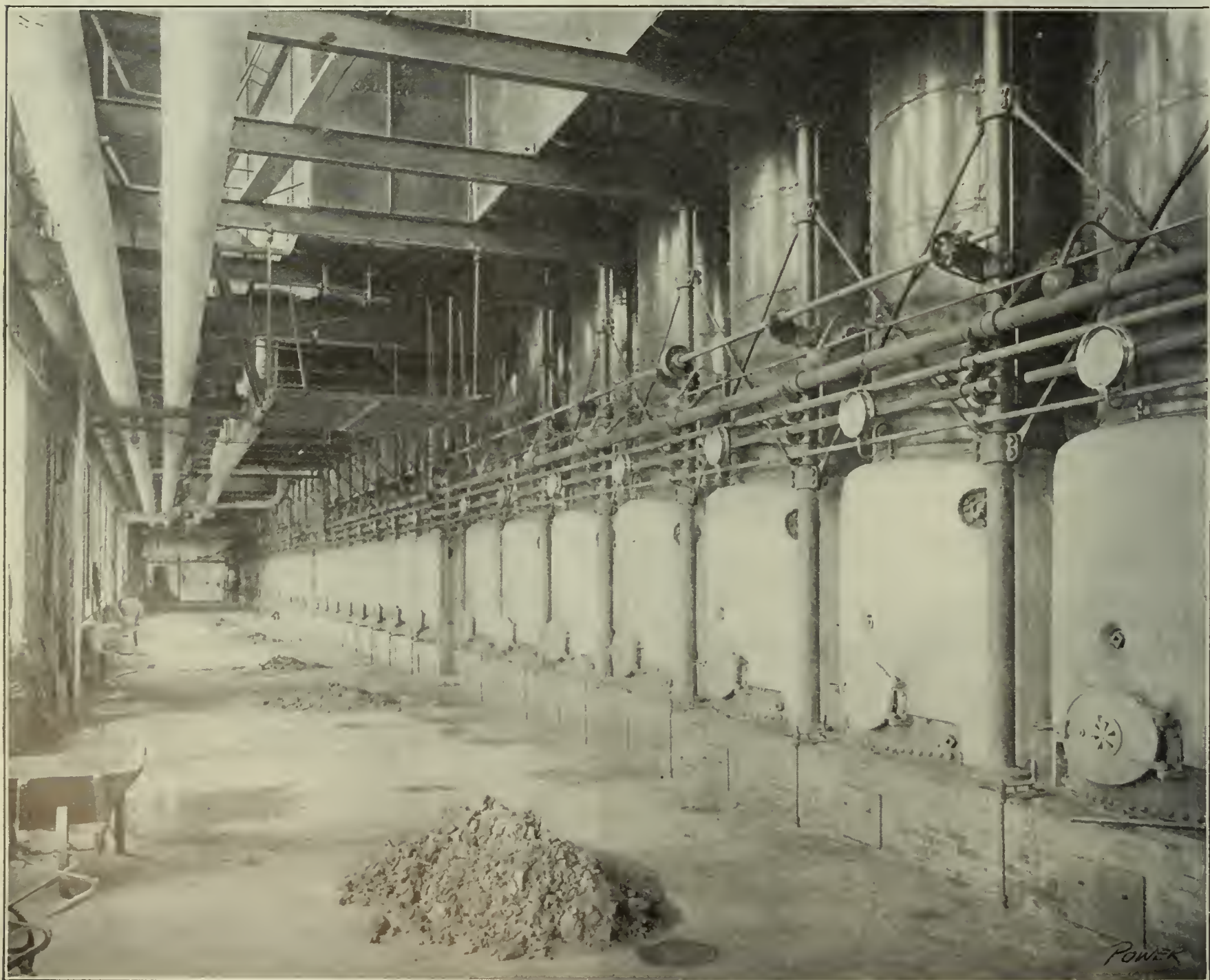
FIG. 1. CLEANING SIDE OF THE MANNING BOILERS. THE HAND LEVER IN FRONT OF EACH BOILER CONTROLS THE AIR SUPPLY IN THE AIR DUCT
