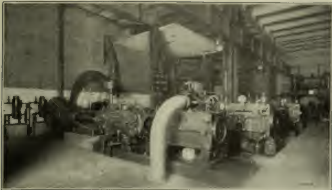
FIG. 14. MAIN AIR COMPRESSORS.
