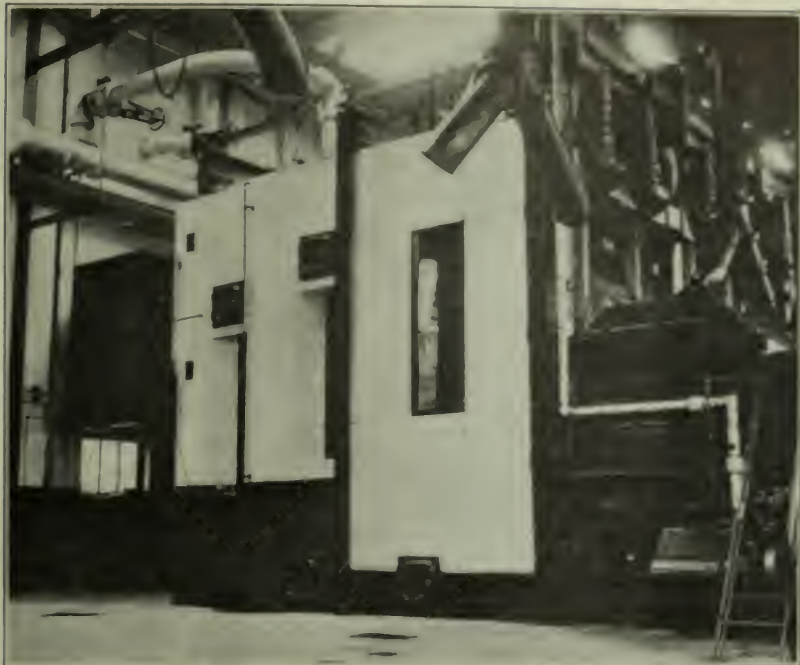
FIG. 2. SHOWING MAGNESIA COVERING ON BOILER SETTING.
