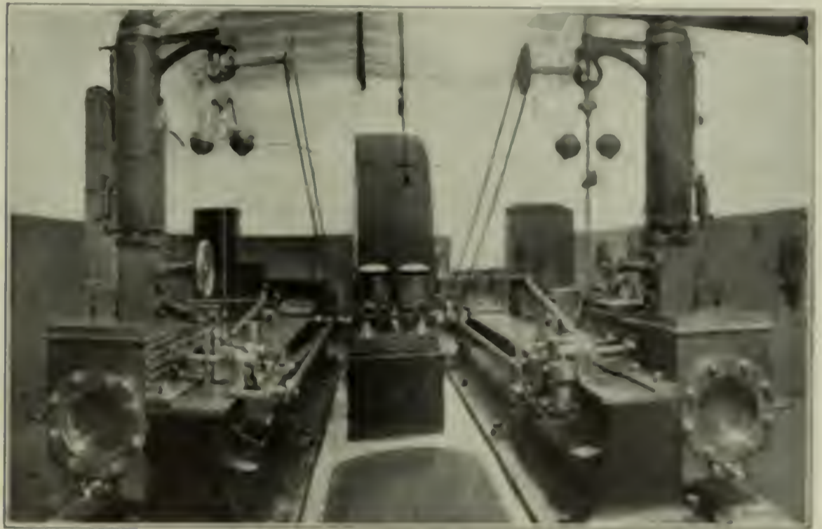
ENGINES AFTER 44 YEARS OF SERVICE
