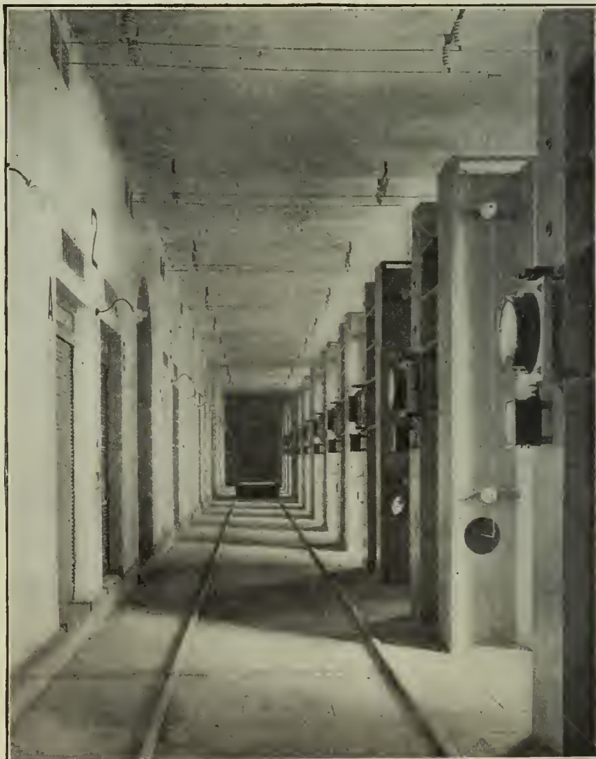
FIG. 7. PASSAGEWAY BETWEEN TRANSFORMER STALLS AND SWITCH STRUCTURE
