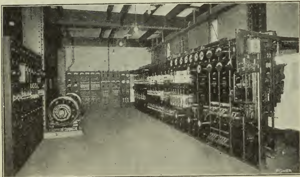
FIG. 1. SERVICE SWITCHBOARD, ALARM SWITCHBOARD AND EXCITERS
