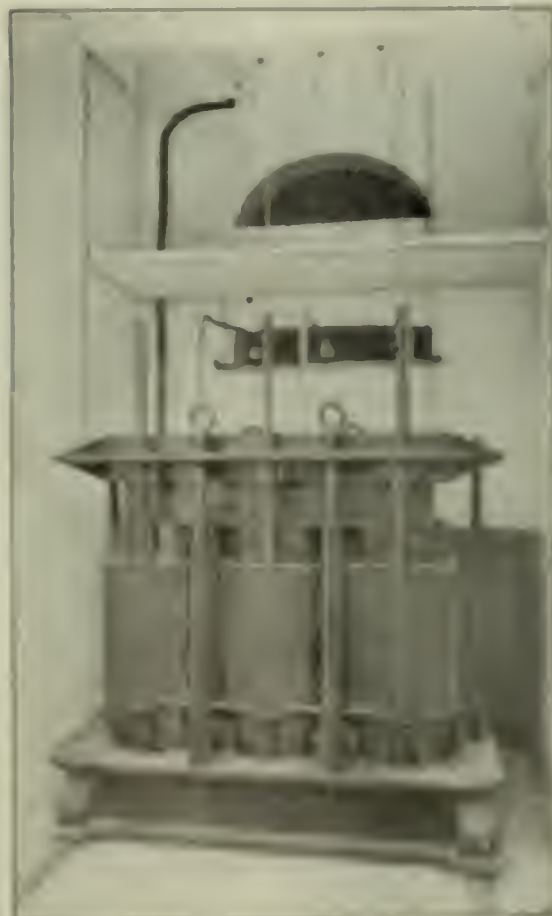
FIG. 4. TRANSFORMER MOUNTED ON WHEELS
