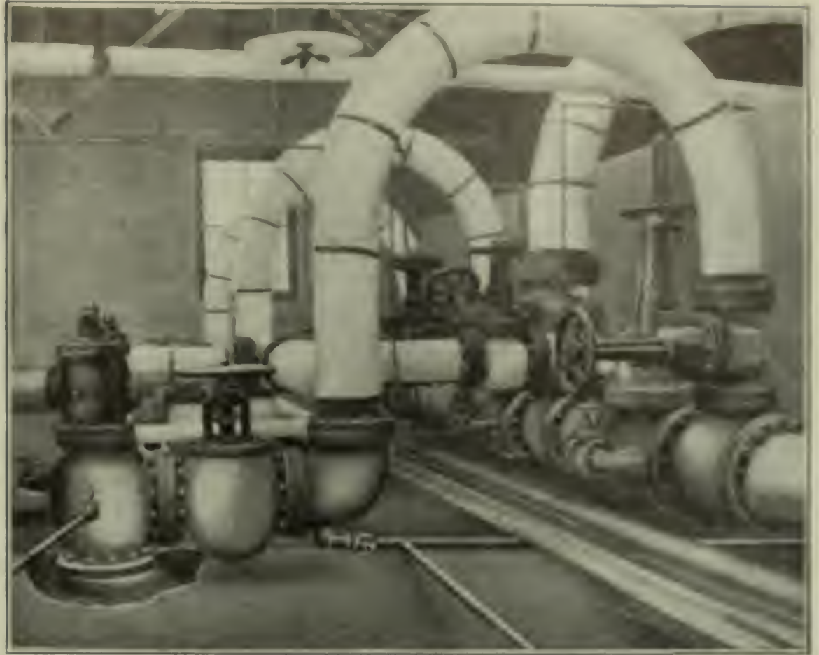
FIG. 2. PIPING OVER THE BOILERS
