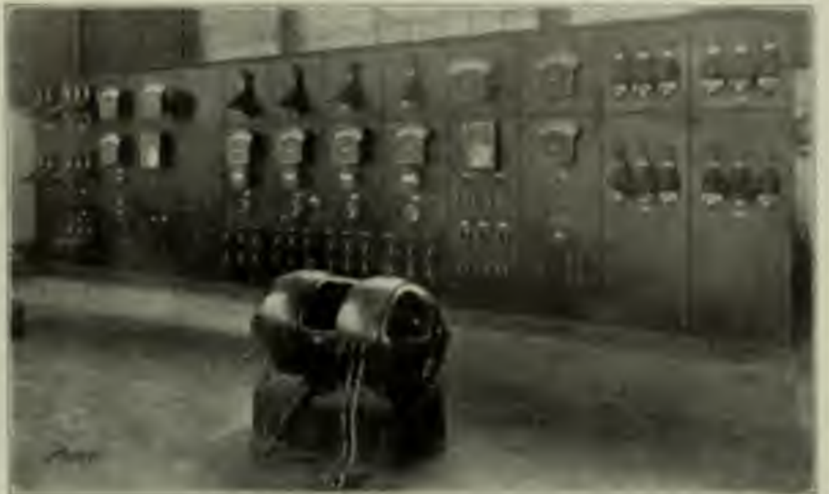
FIG. 3. SWITCHBOARD AND ONE OF THE BALANCING UNITS
