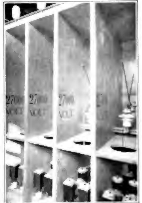
FIG. 5. PART OF SWITCHBOARD
