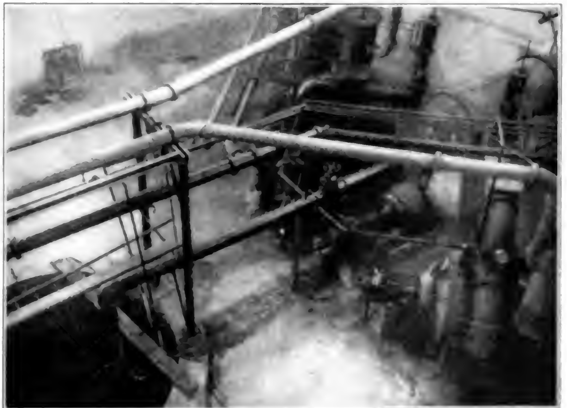
FIG. 9. LOOKING DOWN AT THE BOILER
