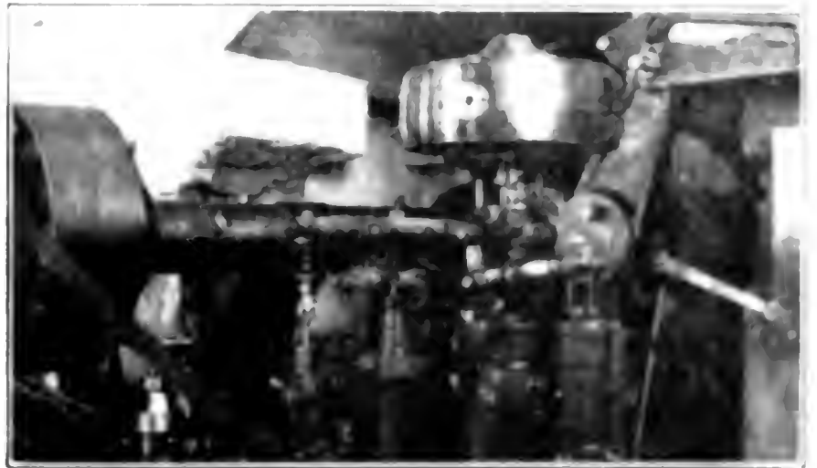
FIG. 8. MOTOR-GENERATOR SET IN NEW WAUSAU PLANT
