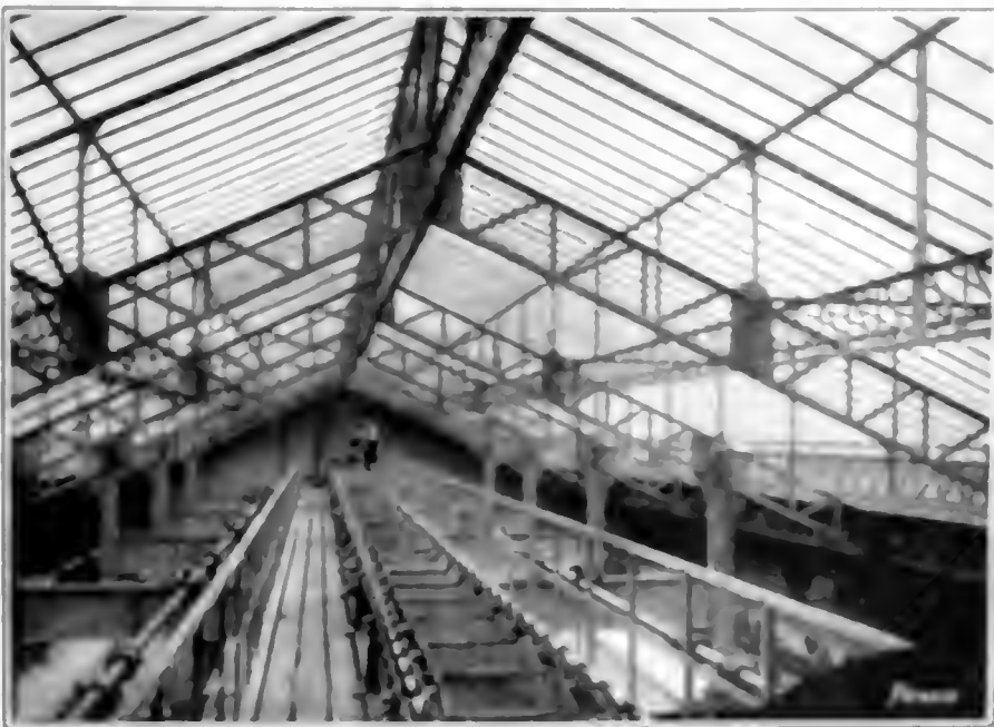
FIG. 5 CONVEYER OVER BOILERS
