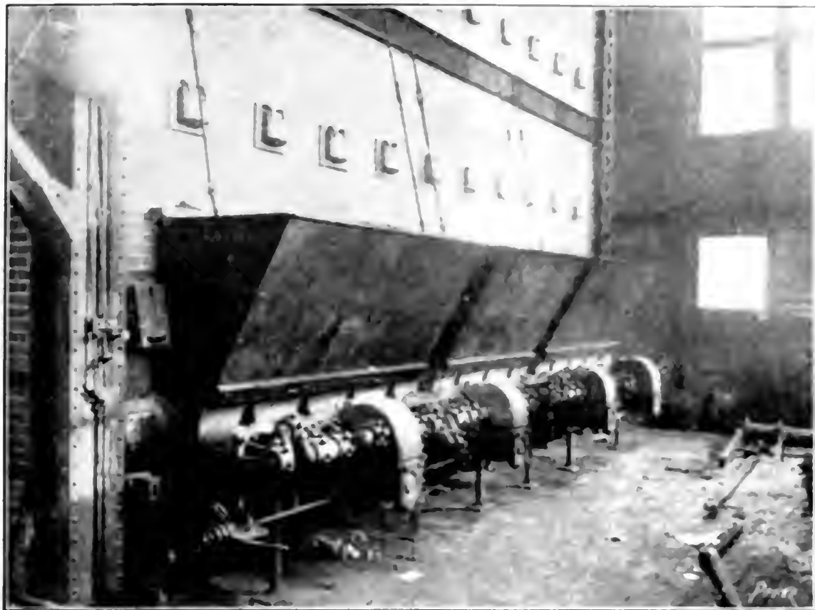
FIG. 2. FRONT OF BOILERS SHOWING STOKER
