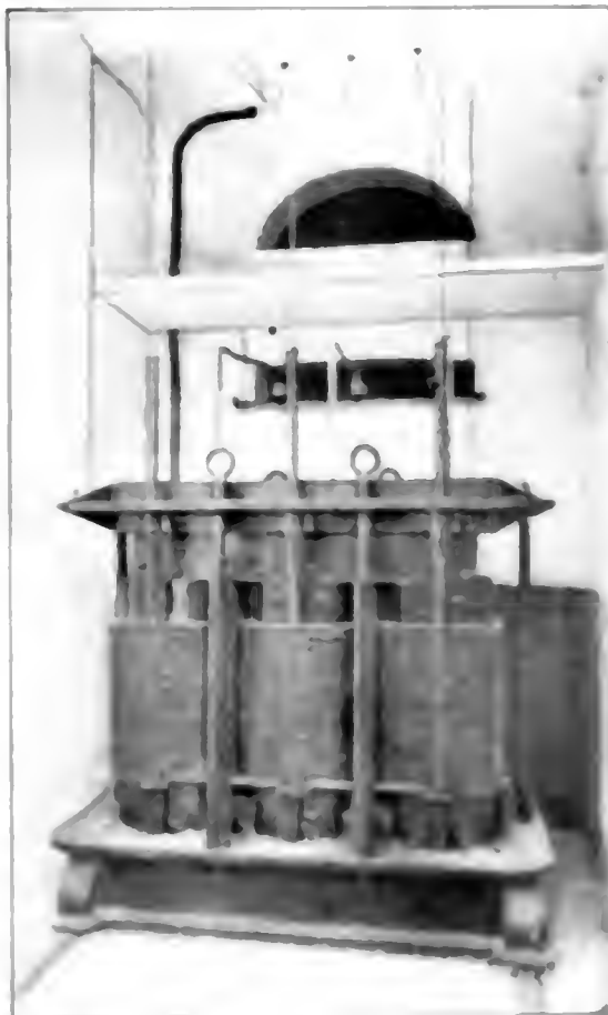
FIG. 4. TRANSFORMER WITH MAXIMUM CURRENT RELAY
