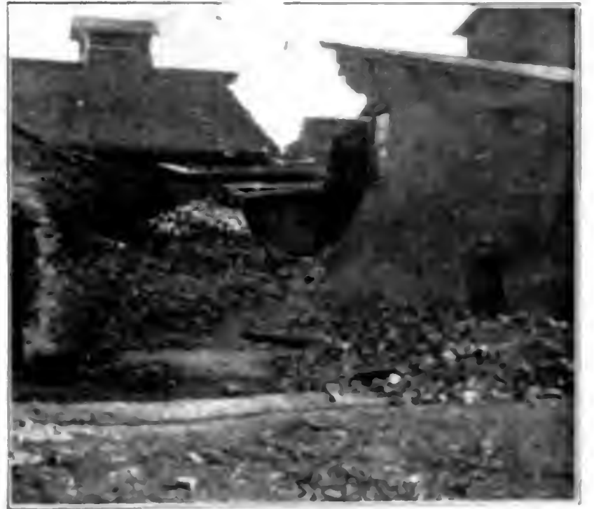
FIG. 3. CRUMBLING BRICKWORK AND BRICK WALL
