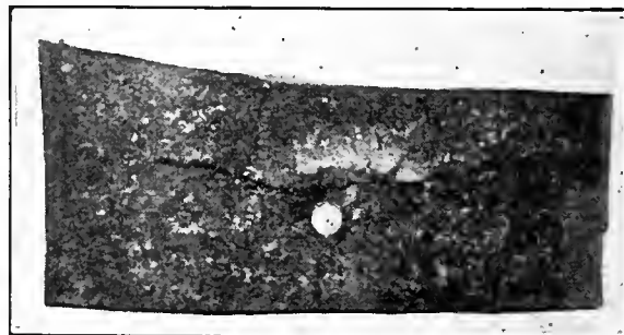
CRACK IN BOILER SHEET
