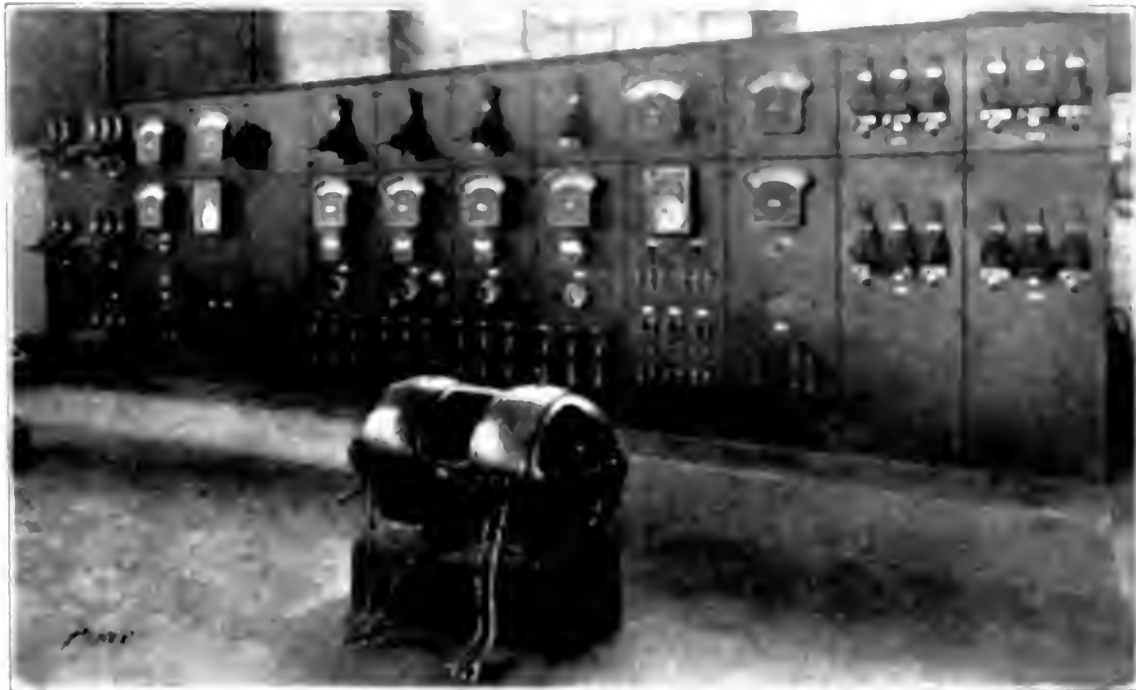
FIG. 3. SWITCHBOARD AND ONE OF THE BALANCERS IN THE BOILER ROOM.
