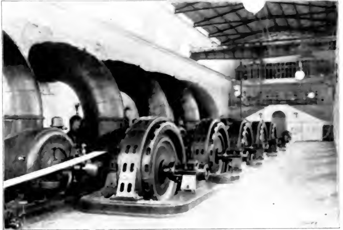
FIG. 3. TURBINE ROOM WITH SWITCHBOARD (COURTESY OF ONEIDA)
