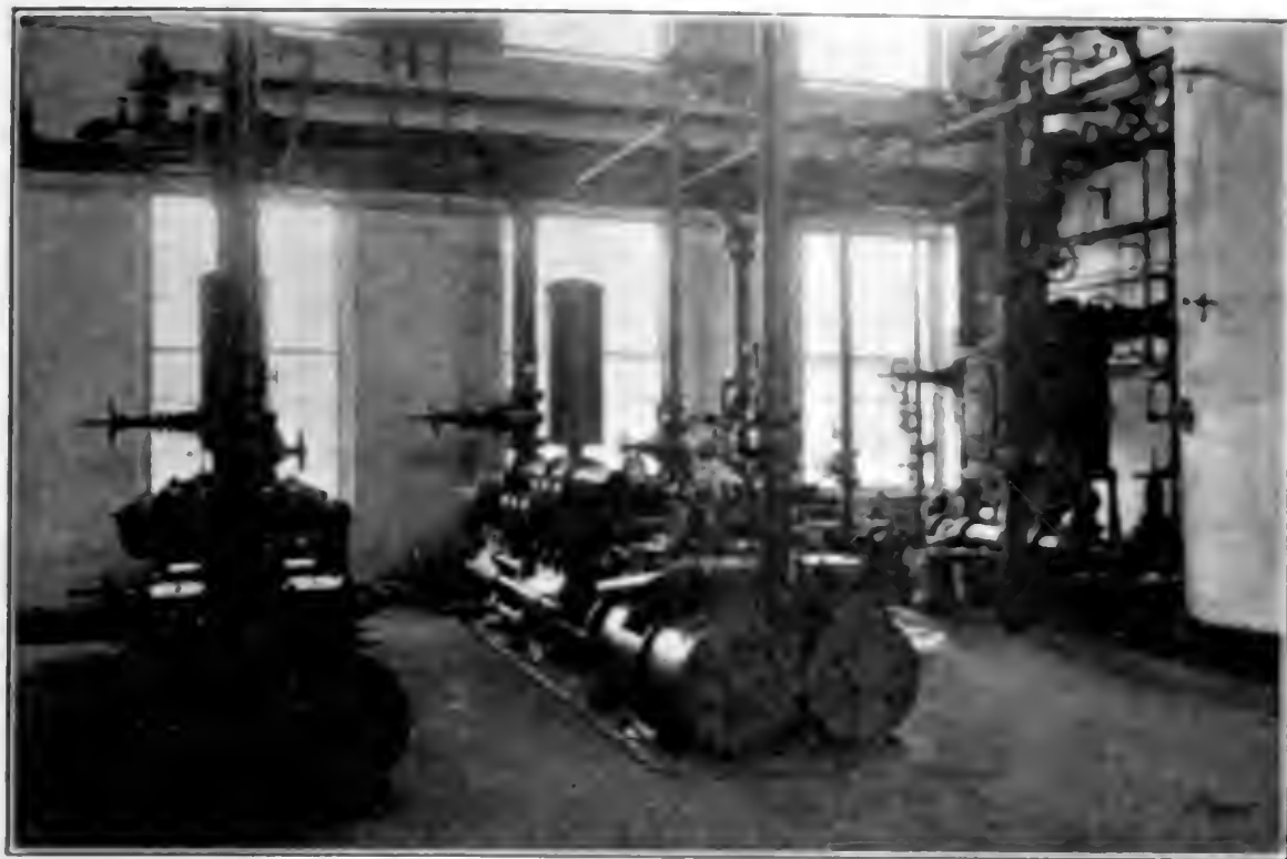
FIG. 8. PARTIAL VIEW OF THE PUMP ROOM
