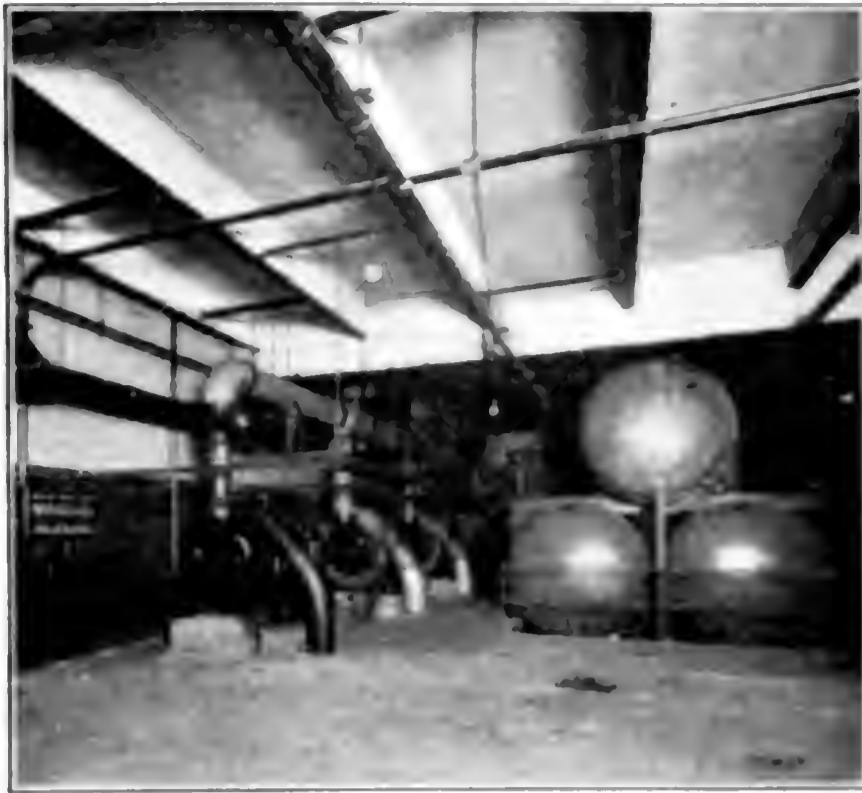
FIG. 5. MAIN HEATERS AND CIRCULATING PUMPS
