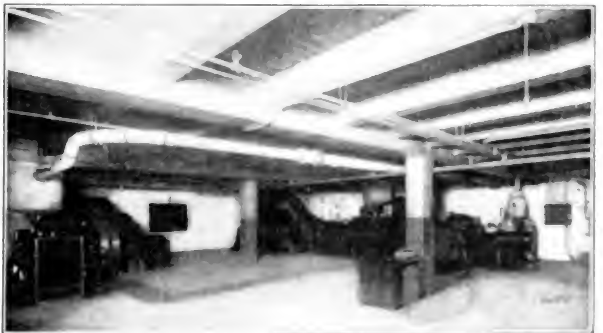
FIG. 4. ENGINE ROOM, SHOWING LARGE RECEIVERS
