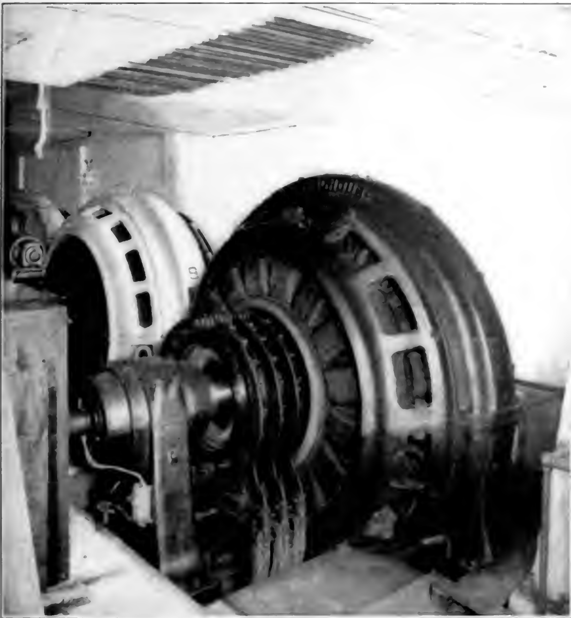
FIG. 4. ONE OF THE SYNCHRONOUS-REGULATOR CONVERTERS.
