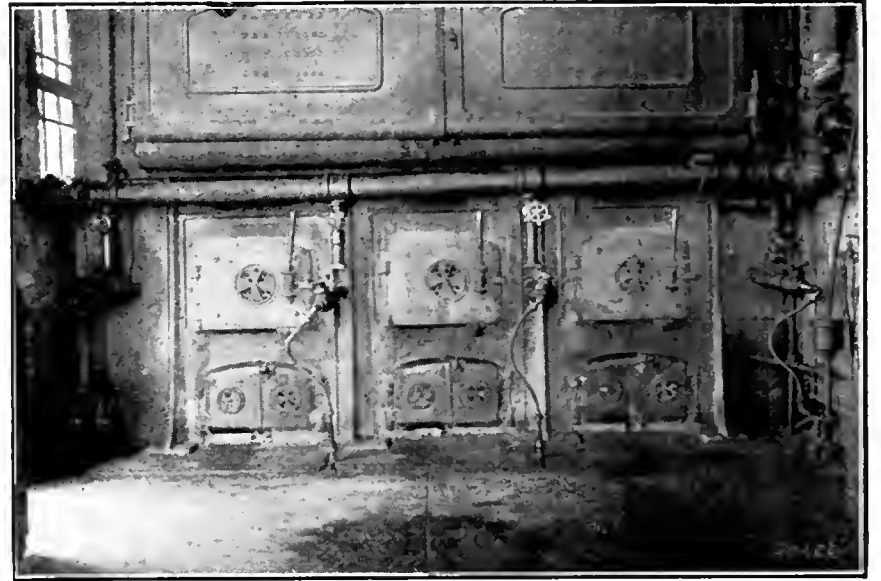
FIG. 3. BURNER PULLED OUT READY TO BURN COAL IN THE FURNACE
