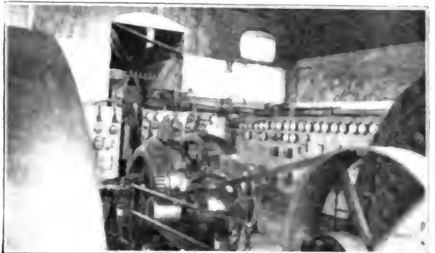
FIG. 6. NEW WAUSAU PLANT
