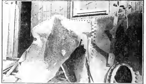
FIG. 2. THE TUBE SHEET. FIG. 3. THE REAR CIRCULAR SHEET NEAR RAILWAY TRACK. FIG. 4. CLOSE VIEW OF PITTED SHEET
