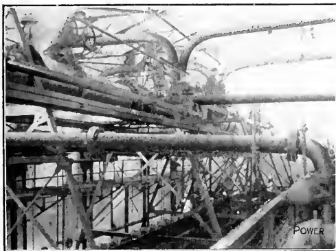
FIG. 2. THE WASTE OF STEAM IN THE AVERAGE MINE PLANT IS DUE LARGELY TO BARE PIPES, LEAKING JOINTS AND WORN ENGINE VALVES AND CYLINDERS
