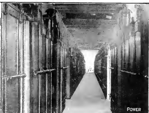
FIG. 16. AISLE BETWEEN REMOTELY CONTROLLED OIL SWITCHES
