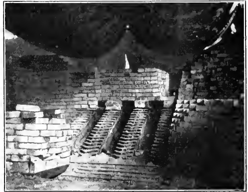
FIG. 4. FURNACE AND STOKER SERVING TWO RETURN-TUBULAR BOILERS
