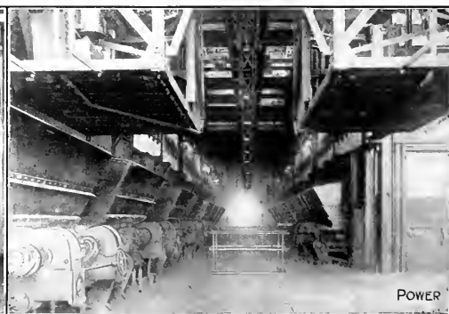
FIG. 6. NEW BOILER ROOM
