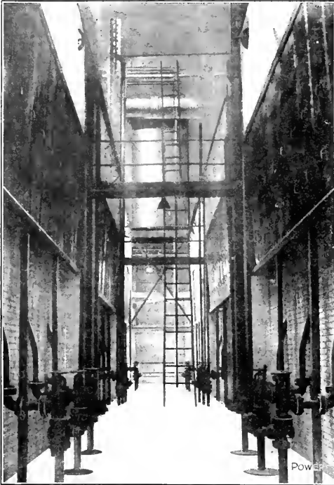
FIG. 7. VIEW AT REAR OF THE BOILERS
