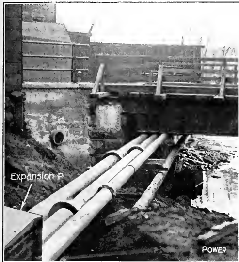
FIG. 3. TWO STEAM LINES RUNNING UNDER A BRIDGE
