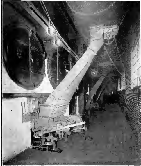
FIG. 3. A THREE-RETORT UNDERFEED STOKER SERVING TWO 72-IN. RETURN-TUBULAR BOILERS
