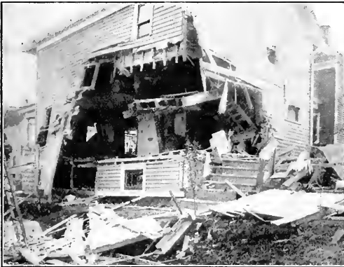
FIG. 1. CONDITION OF PREMISES AFTER EXPLOSION
