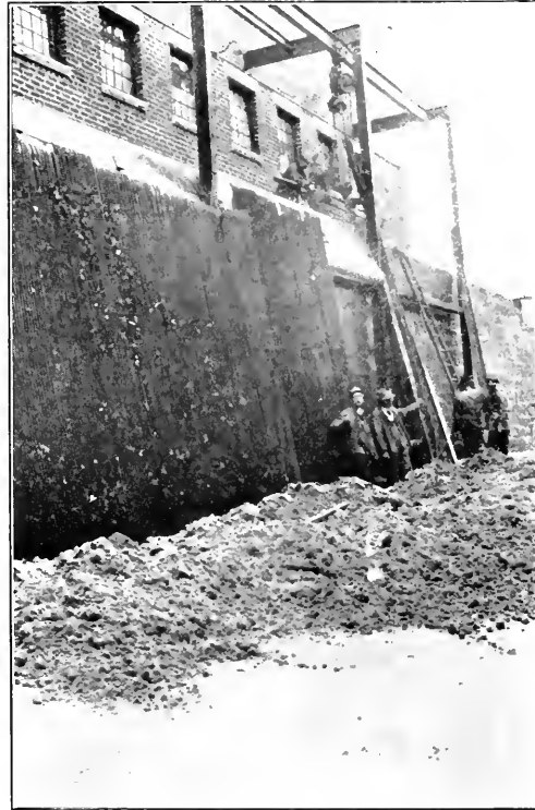
DIRT AT THE INTAKE SCREENS
