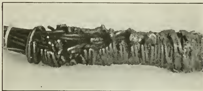
CONDITION OF SPLICE AFTER BURNOUT
