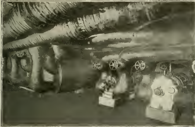
FIG. 5. CENTRIFUGAL BRINE PUMPS AND BRINE COOLERS
