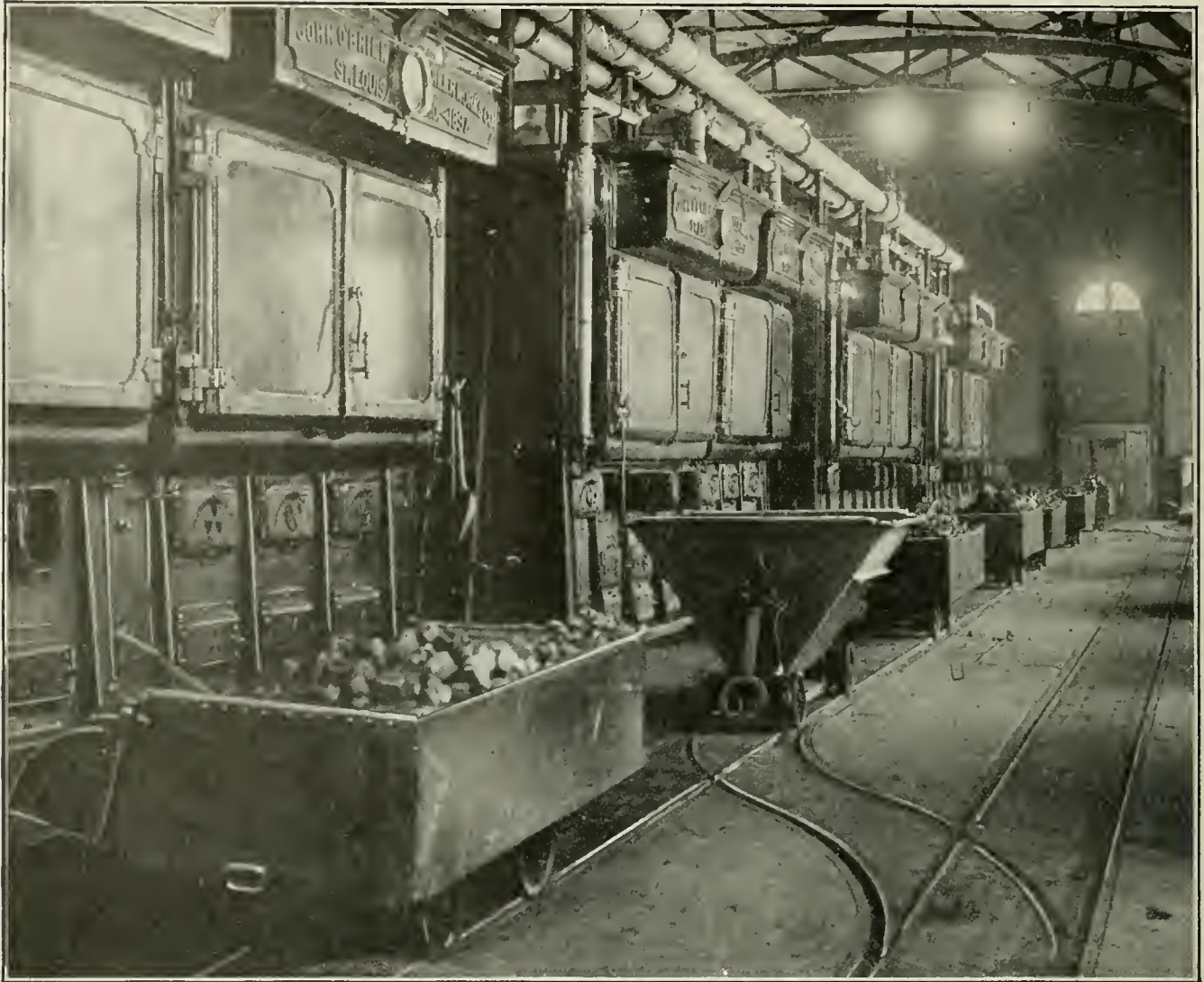
FIG. 1. INTERIOR VIEW OF THE PRESENT BADEN STATION BOILER ROOM
