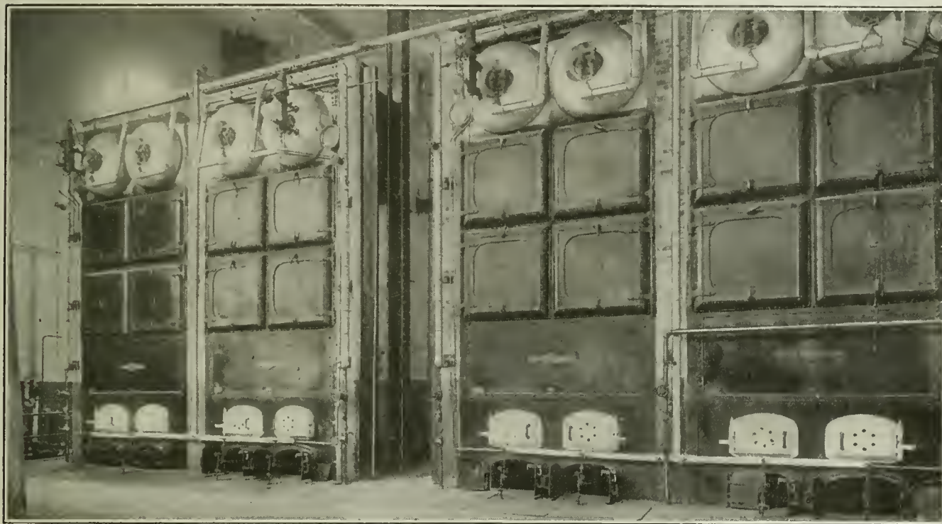
FIG. 2. OIL-BURNING BOILER ROOM, TAMARACK MILLS
