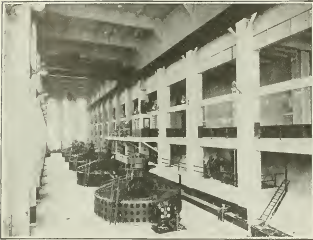
FIG. 5. 90,000-HP. GENERATORS—COOSA RIVER INTERIOR VIEW LOCK NO. 12 POWER HOUSE
